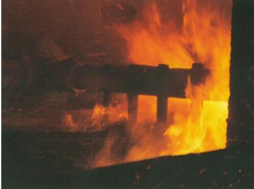
Inside of incinerator
